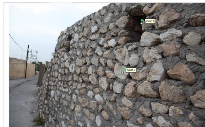
Figure 2. A wall on the verge of collapsing.
