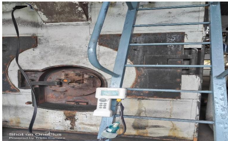
Figure 3: Running boiler performing stack analysis
