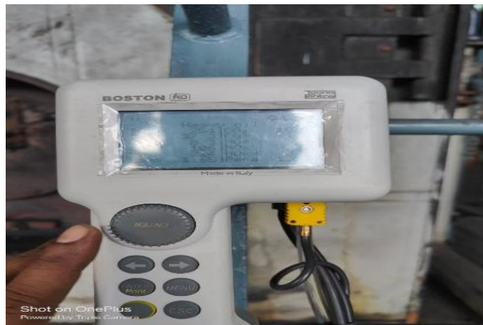
Figure 2: Gas analyzer connected to boiler stack
